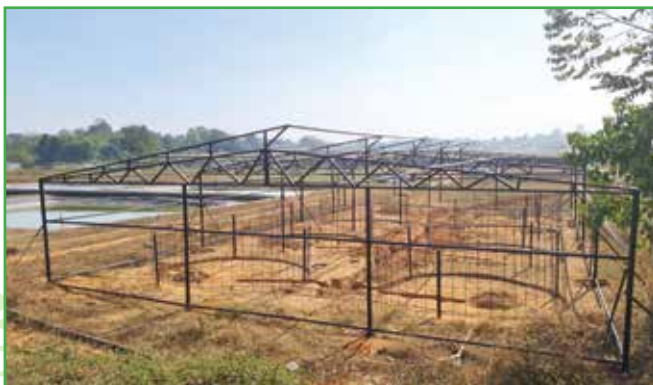
Biofloc tank facilities
