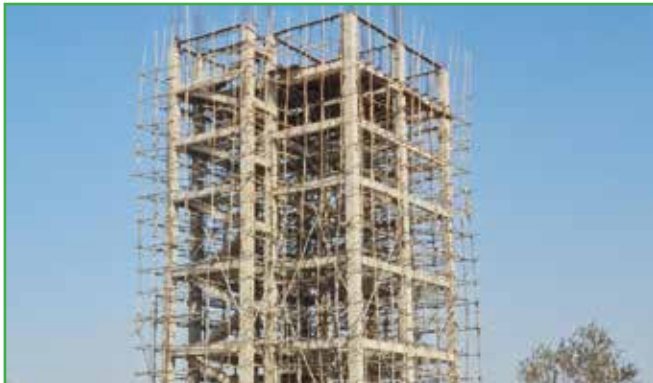
Overhead water tank
