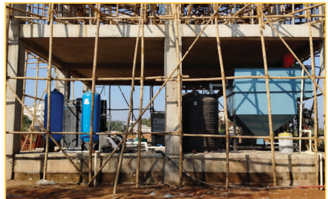
Water treatment plant at Farm A
